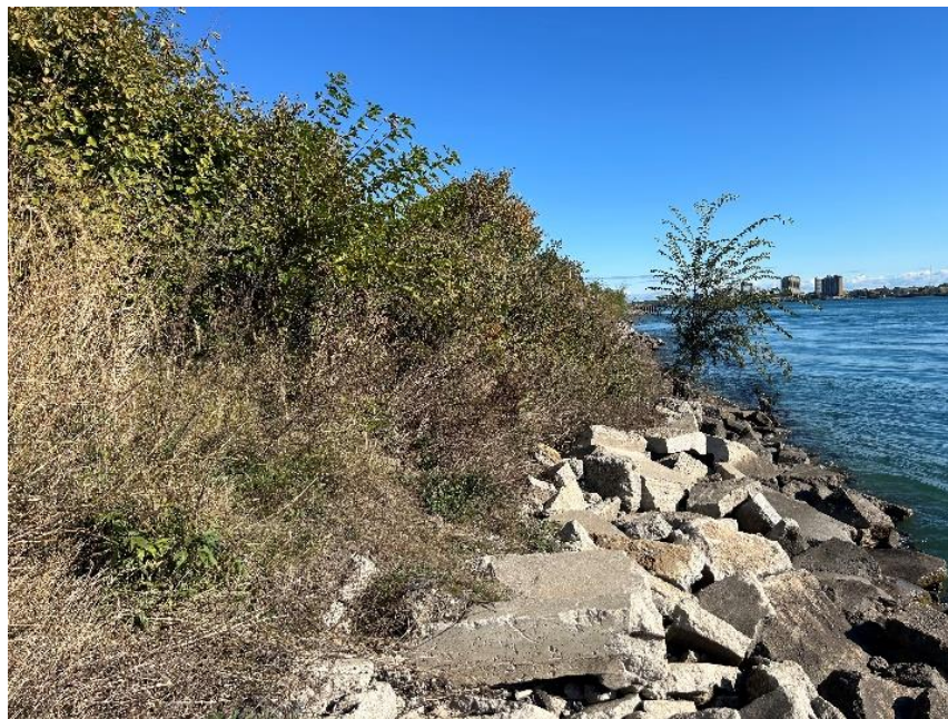
Figure 8. Cement riprap lines the shoreline edges helping to prevent erosion from large waves and fast river currents while also providing habitat for aquatic fish and macroinvertebrates. Native plants, as shown in this photo, have large root systems that hold soil in place and maintain the integrity of the shoreline. L. McFadden.
