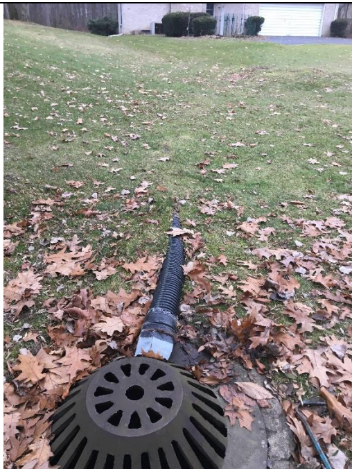
Plastic PVC drain from 482 Whippers LN connected to Back Yard CB Beehive. No flow.
