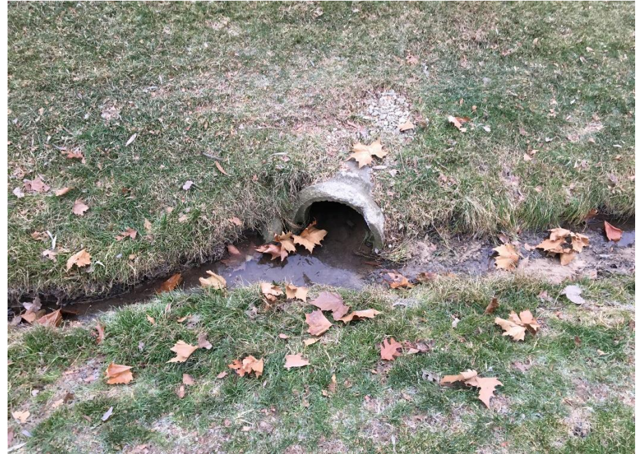
Drainage Ditch N. of MH 408. Flow is clear. Inlet pipe in ditch connected to MH 410.
