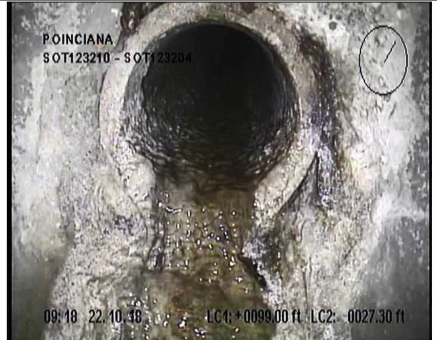
6" Clay Tile Tap at 102.1 ft. S. of MH SOT123210 under driveway for 21208 Poinciana
