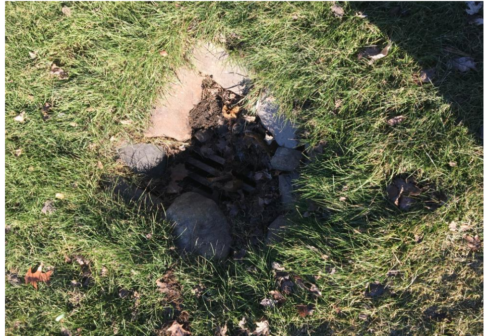
Dover 1 CB located W. of drive at 4810 Dover. Cover buried under landscaping rocks
