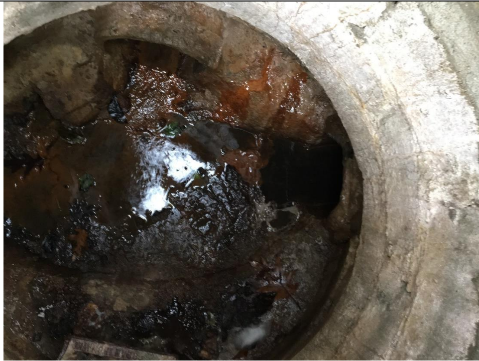
MH 7316. Terminus MH. Connects local drains W.& S. Sewage and animal Feces in MH
