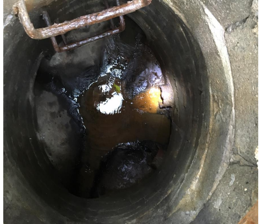
Dover 4 MH in Charring Cross at Dover. Rd rain Inlets E & W. Inlet. N with flow. Sampled
