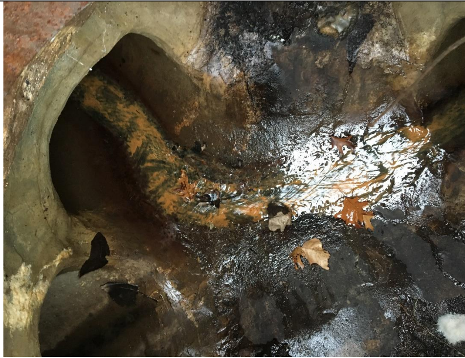
MH 407 flow from N. Rd drain inlet E. is dry w/ animal feces in MH. Sampled
