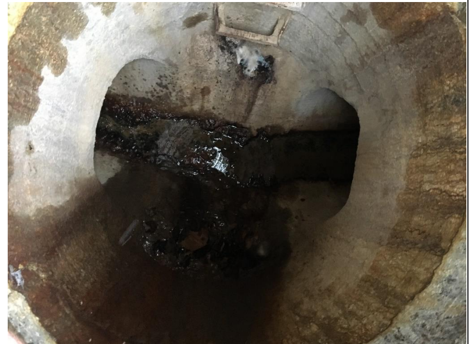
MH 410 – Connecting MH CB B 13378 to drain going E. Animal feces in MH. Sampled
