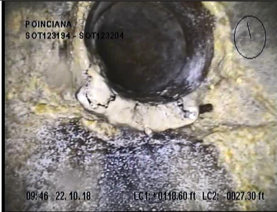
6 "Clay Tile Tap 119.0 ft. N of MH SOT123194 between 21120 & 21130 Poinciana
