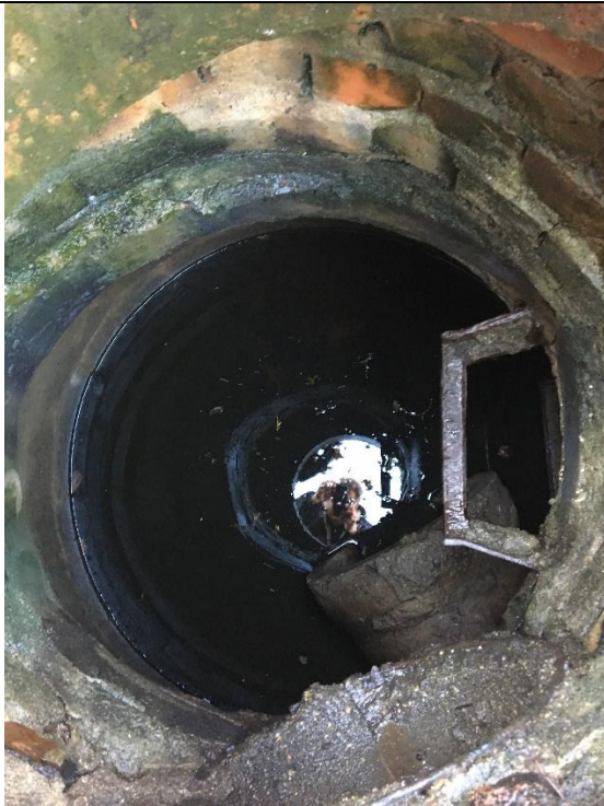
MH on Hunt Master. Connects Rd drain ditches to drain. Water in CB sump. Sampled
