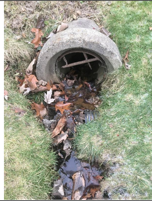
Inlet to CB 13369 w flow from drainage ditch to the W. Flow is clean
