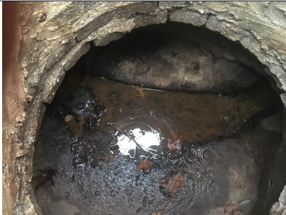
MH 7318 Connected to MH 407. Animal Feces on MH floor and channel. Sampled
