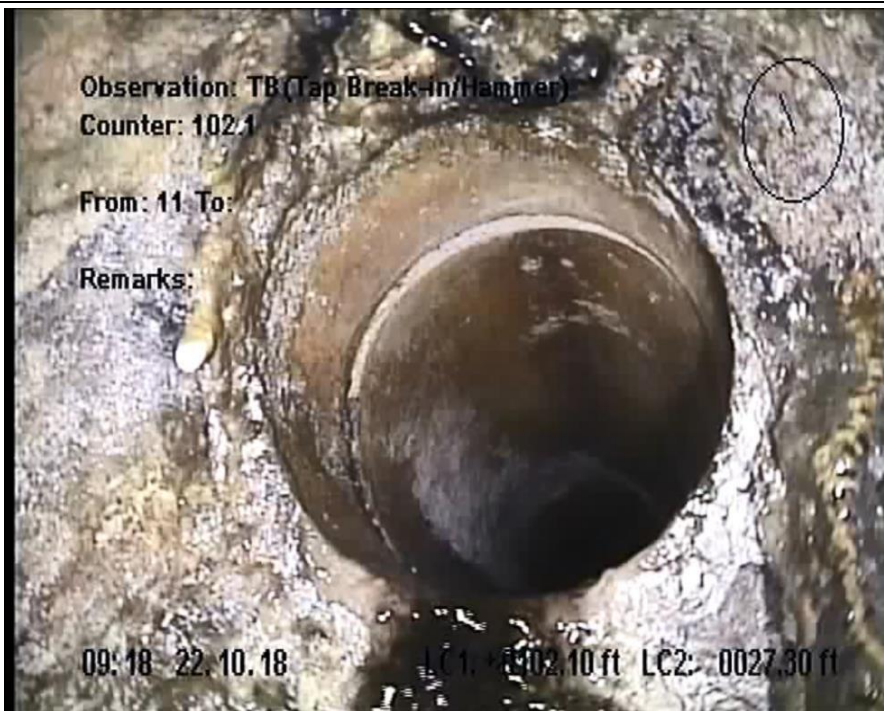
6" Clay Tile Tap 99 ft. S of MH SOT123210 between 21207 and 21121 Poinciana active flow
