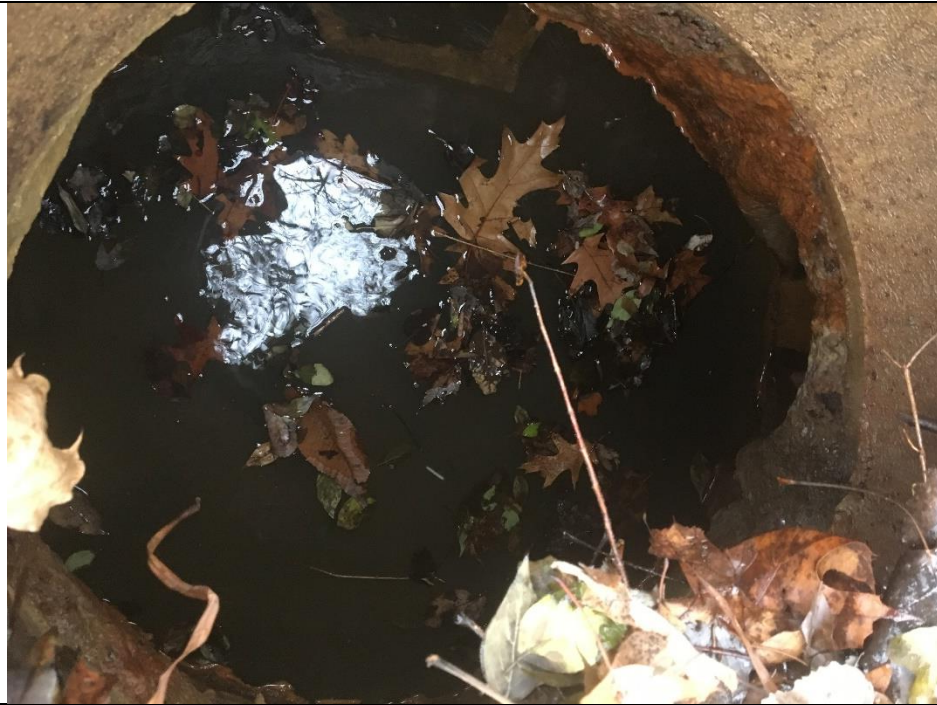
CB 13369 connected to MH 7317. Inlet flow from ditch line W. Looks clean. Sampled
