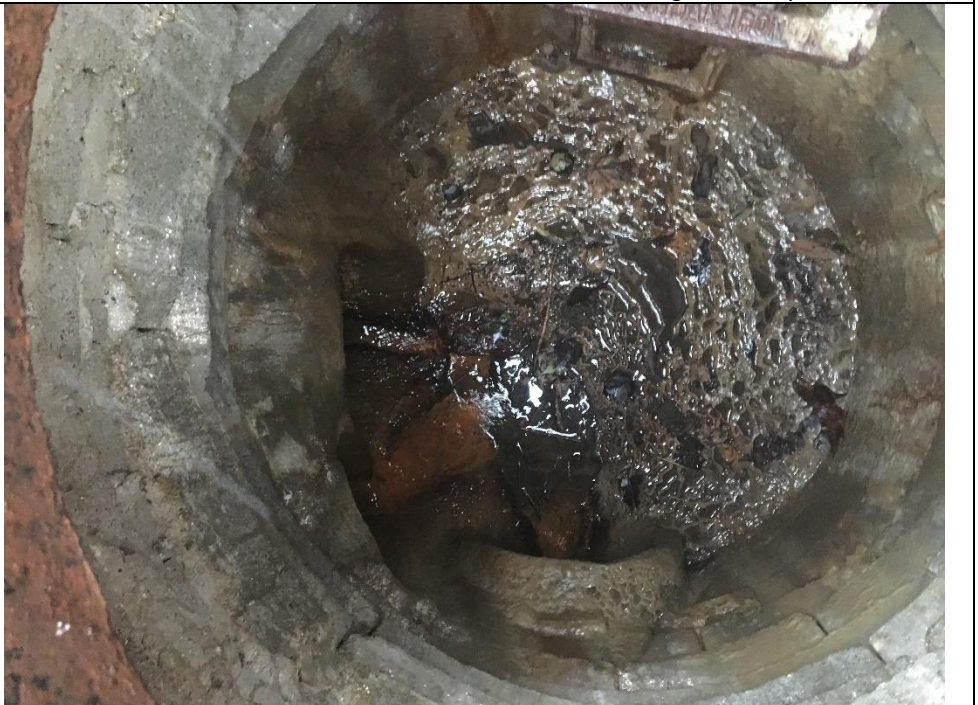
MH 7317. Elbow from W. to S. Possible sewage in MH. Sampled. Connected CB to the S.
