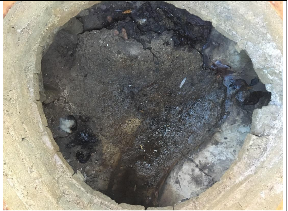
local storm MH for connected Rd drains on E. side of Charring Cross. Dry w animal feces
