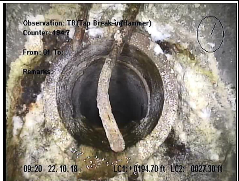
6" Clay Tile Tap 194.7 ft. S. of MH SOT123210 @ 21185 Poinciana w active Flow
