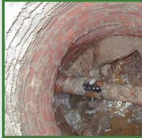
Broken sanitary sewer
