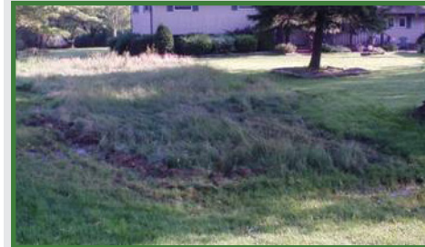
Overgrown septic field
