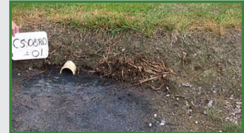
Cheater pipe from septic field
