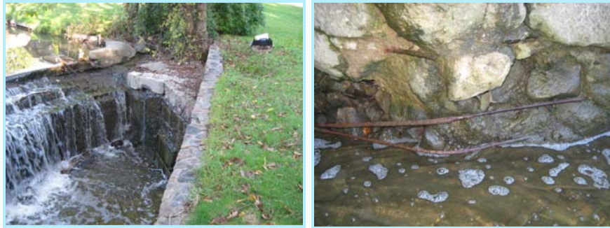
Existing Conditions: Failing Dam
